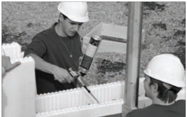
Students from the MSU-Great Falls College of Technology work on building a house that will be sold by NeighborWorks to a family that makes less than 80 percent of Cascade Median Income. COT students helped on the job site for NWGF's Mutual Self Help families, who build their own homes, but this is the first time the COT faculty and students are building an entire home in conjunction with NWGF.
